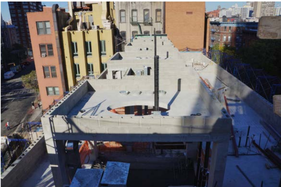
Looking down at the unfinished Sullivan townhouses from the 5th floor terrace
